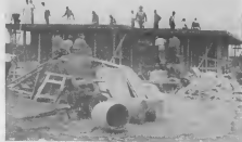
Perhaps the latest method for building homes is introduced to Aruba by Jorge de Castro of Oranjestad. This house is being "poured" using a cement mixture which has been chemically expanded into a lightweight building material. Forms are placed and then the mixture is pumped in by hoses, forming walls and ceilings. The resulting home is economical and sturdy. Its structure is fire-proof, vermin-proof, and sealed against weather.
